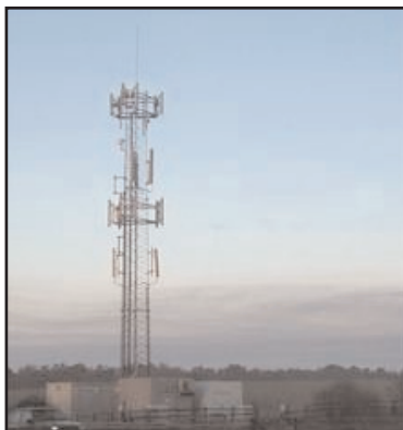
Typical cell site
